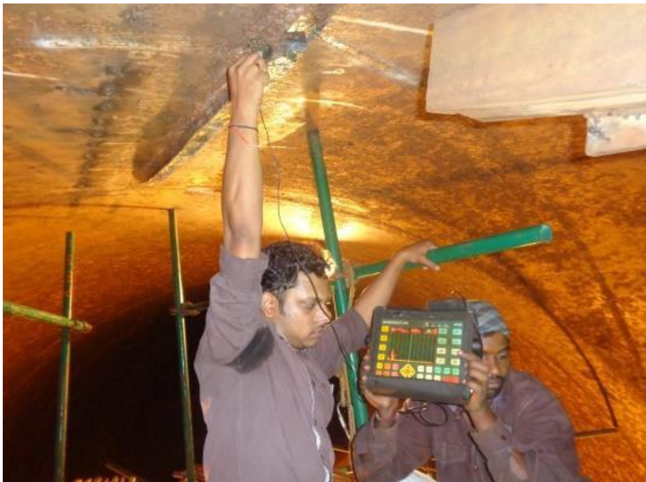
11C- Lamination found in UT at Chainage 18.5 – 19.0.
