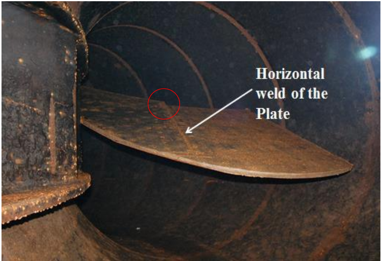
Fig.3[1].Part of Sickle Plate found in Spiral casing of Unit 2. Geometric Stress raiser seen at the location marked with Red Circle .
