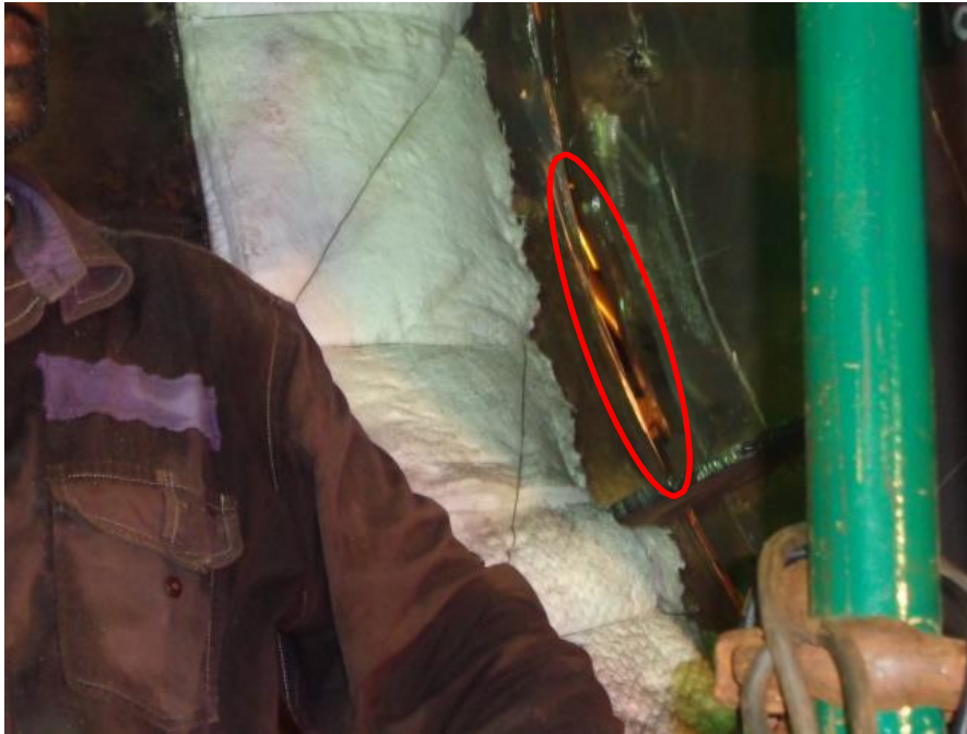
Fig.12A-Transverse cracks removed by grinding., resulting in uneven root gap.
