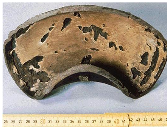
Figure 1-2: Erosive-corrosive effects on elbows of flowlines
