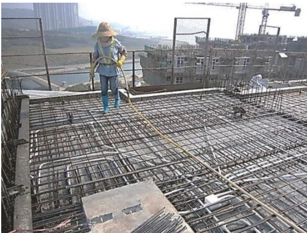
Fig. 40 Laying of electrical conduits and fabric reinforcement on top of semi-precast slab
